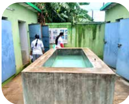
Built 22 integrated sanitary toilets for women and children and 2 public toilets to reduce the open defecation problem and maintain a clean and hygienic community environment.
